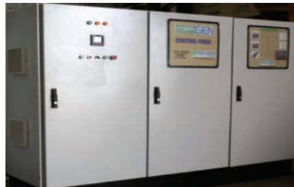
Fig. 23 b: Power conditioning unit
