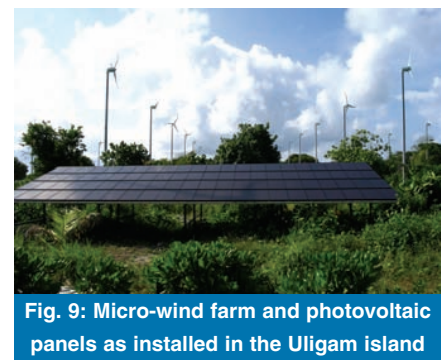
Fig. 9: Micro-wind farm and photovoltaic panels as installed in the Uligam island
