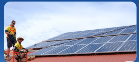
Regen Power 10 kW Solar PV System installation at Saint Mary Church, Calamvale
