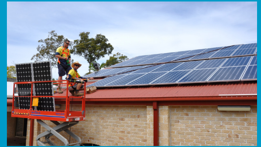
System installation by Acsel
