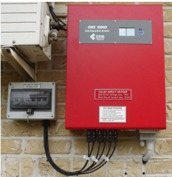
11 kW, 3-phase CMS inverter
